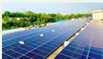
Pahartali Textile & Hosiery Mills 1.32MW Rooftop Solar
